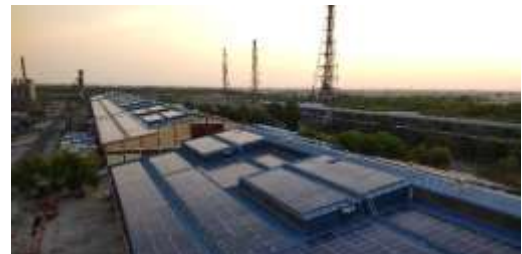
5.76 MW Rooftop project of GAIL- SECI was the PMC
