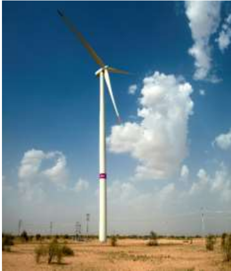
Wind Turbine in a 250 MW Project under SECI tender
