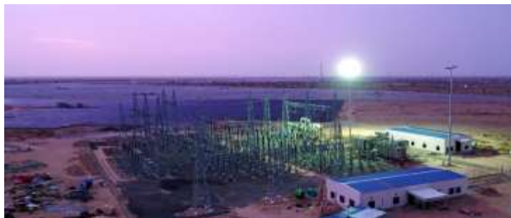
390 MW Solar Project under SECI tender
