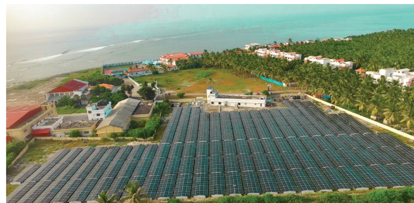
1.7 MW solar power project with a 1.4 MWh battery energy storage system in Lakshadweep
