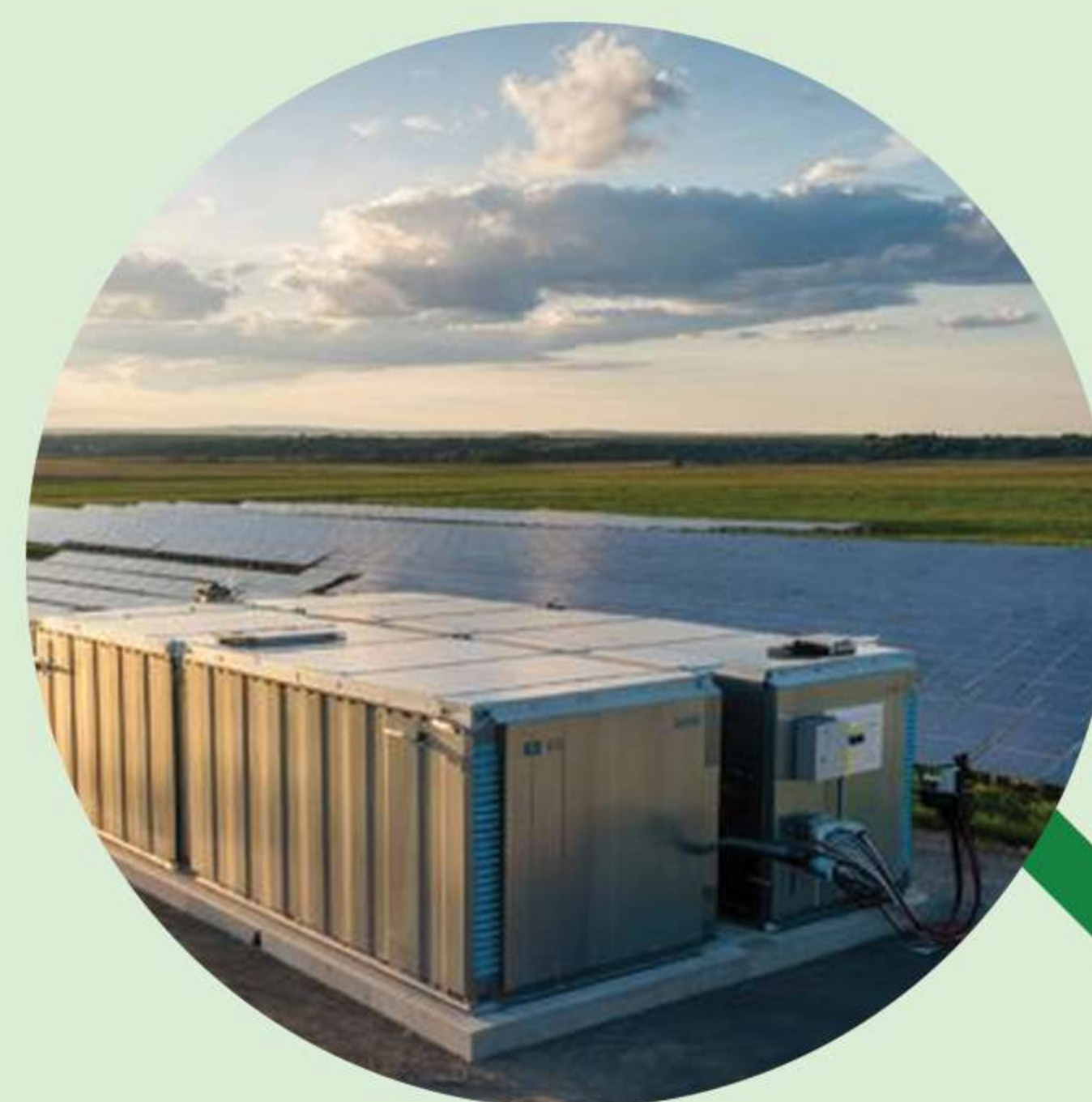
Hybrid & Battery Energy Storage System
