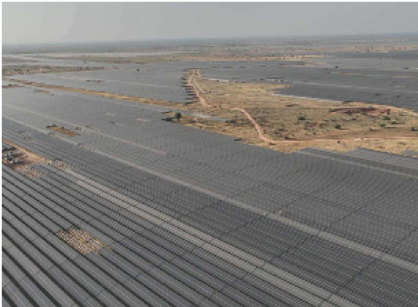
300 MW Solar PV project, Jaisalmer, Rajasthan.
