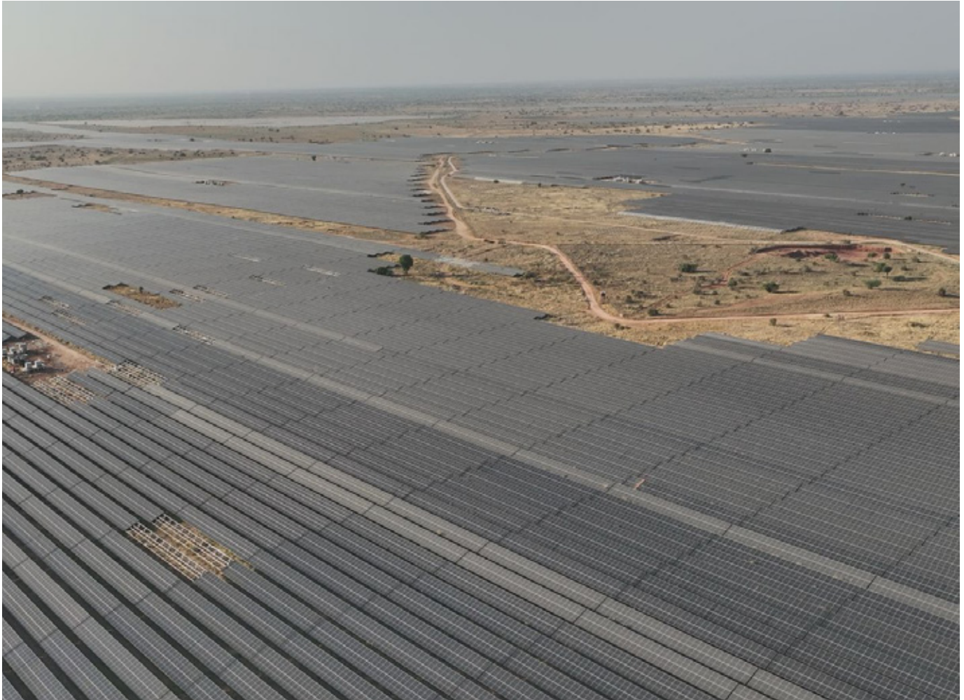
300 MW Solar PV project, Jaisalmer, Rajasthan.
